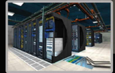
Data Center & Power
